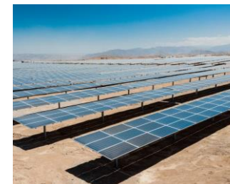
Intipampa (2018) • 40MW - Solar
